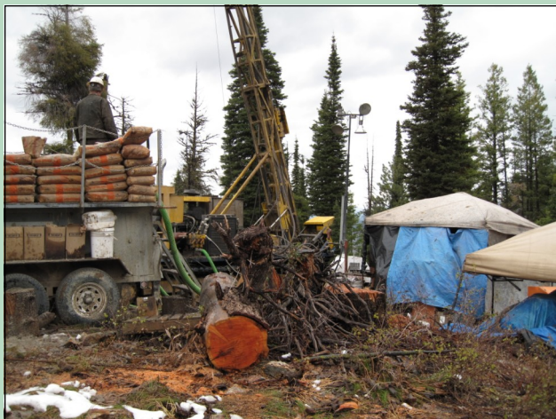
One of many drilling sites at the CuMo prospect mine in Fall 2009.
